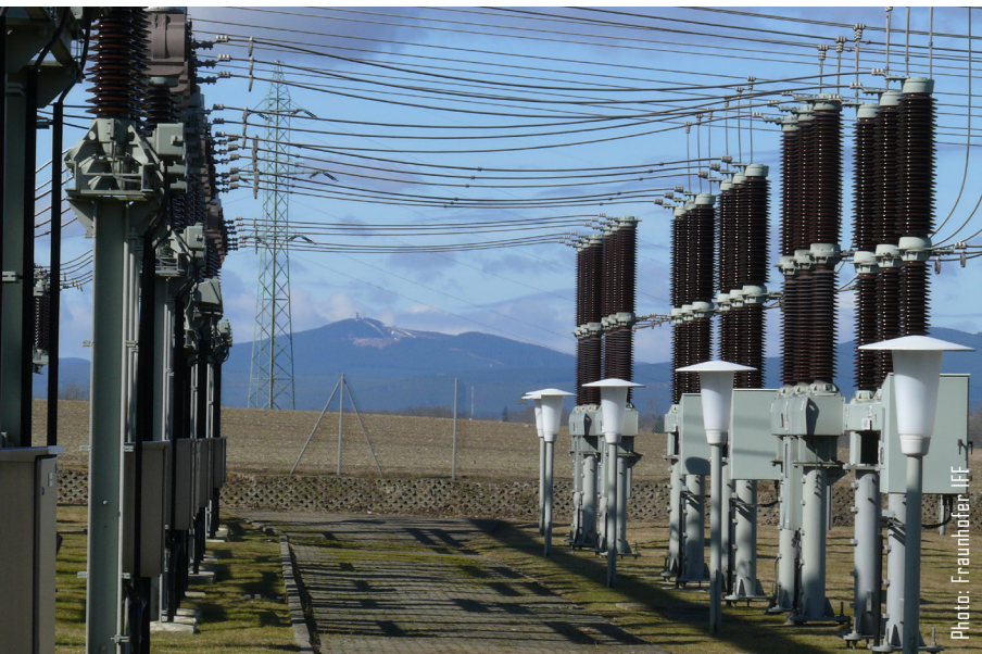
SECVER is determining the actual power flows in the 110 kV high voltage grid in a transformer substation in the Harz test region.
