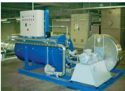
Figure 2: Thermal afterburning modules with exhaust and combustion blowers.
